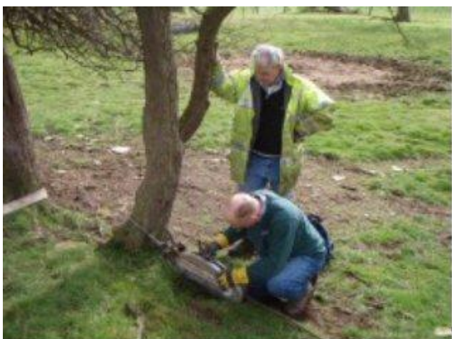
SPECIAL EQUIPMENT IS USED TO PULL UP DEEP OR STUBBORN ROOTS FROM THE CANAL BED
