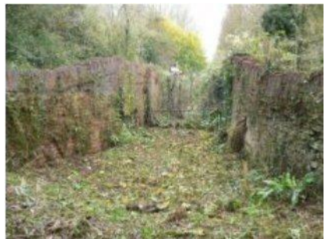
THE 'BEFORE' SHOT - HYDE LANE LOCK - MADE POSSIBLE BY A GRANT FROM WREN.
